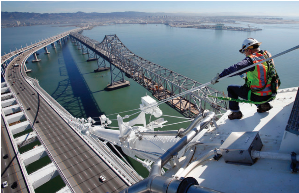
Caltrans bridge engineer Brian Boal prepares to step onto the main cable of the new Bay Bridge on Feb. 21, 2014, in San Francisco. (Karl Mondon/Bay Area News Group)
